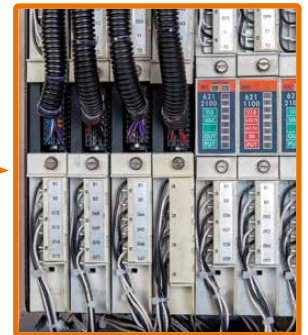
Completed and migrated DCS System
