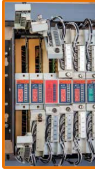
Remove existing Field Wiring adaptors
